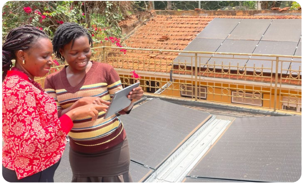
Photo: Lilian Ahimbisibwe and Linda Babirye are monitoring the new solar panels on the office roof in Kampala
